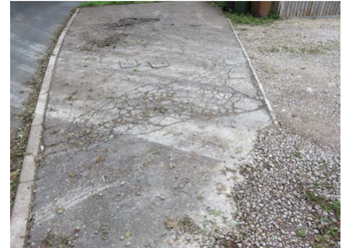
Poor surfacing to a large access splay
