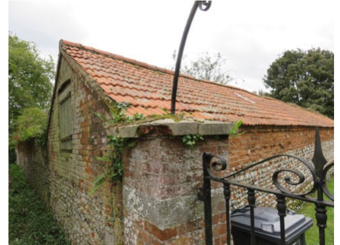
Damage to the capping of the gate pier to the churchyard
