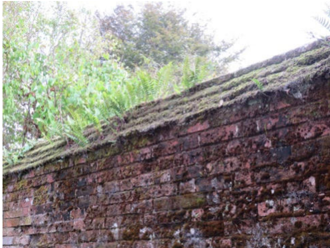
Vegetation growth to a boundary wall near overhanging trees
