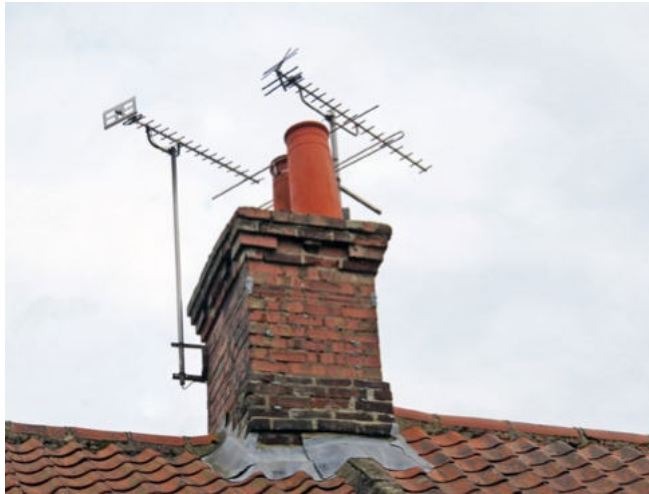
Television aerials and associated supports and cabling detract from the appearance of historic buildings and can cause damage to the historic fabric.
