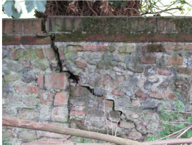
Cracked boundary wall due to tree growth
