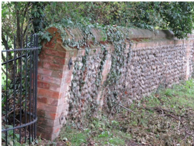
Leaning boundary wall
