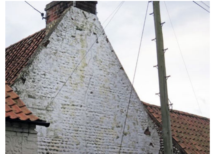
Damp and staining in a gable end fronting the main road
