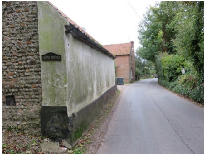
Missing drainpipe and evidence of building being struck by a vehicle on the main road
