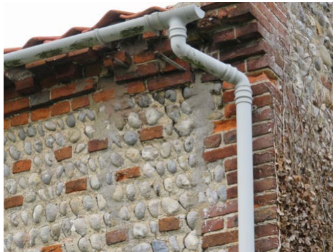
Cracks and cementitious repairs to a building
