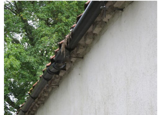
Broken gutters cause water to soak the walls, which leads to deterioration of the fabric
