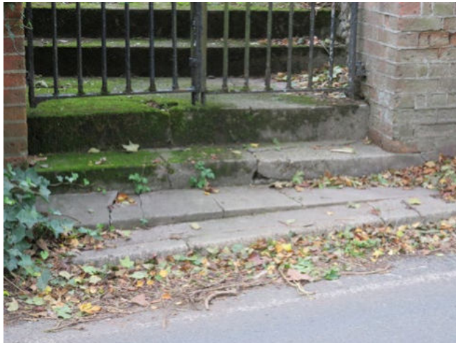
Cracking cementitious screed to steps
