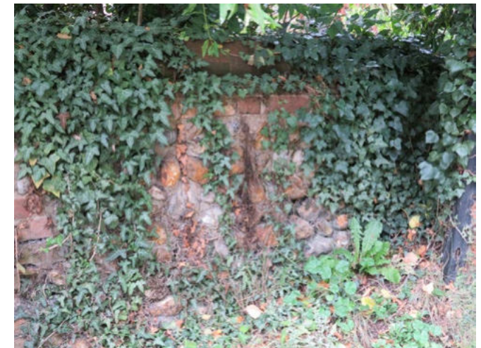
Vegetation growth causing damage to the brick and flint boundary wall
