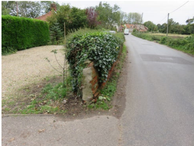
Inadequate termination to the wall with cement render; also ivy growth
