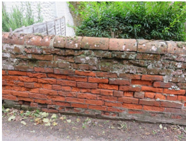
Boundary wall brick decay resulting from proximity to the road
