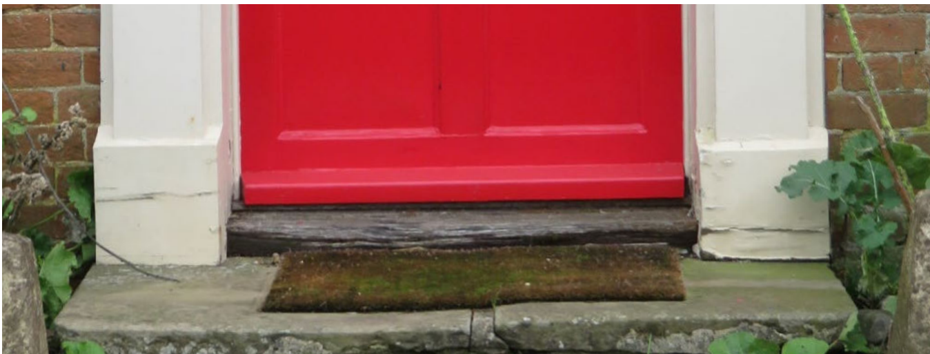
Rotting base to doorcase
