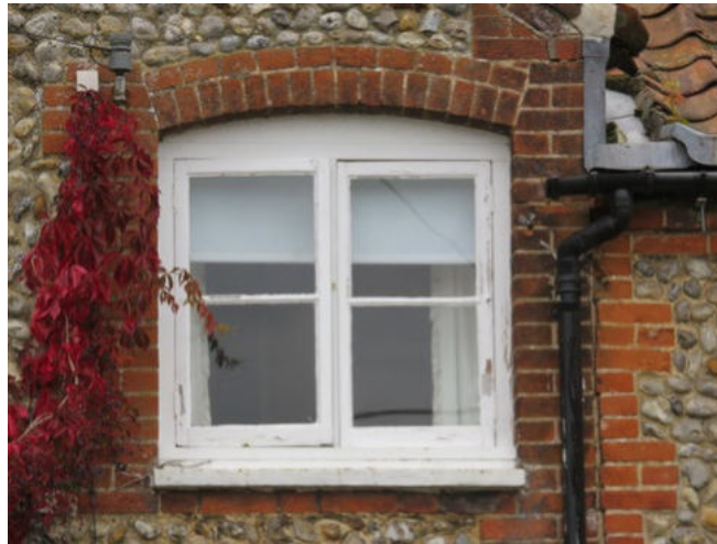
Example of external timber joinery requiring repainting
