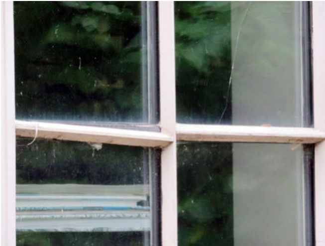
Glazing bar that has come unstuck on a slimline double glazed replacement window
